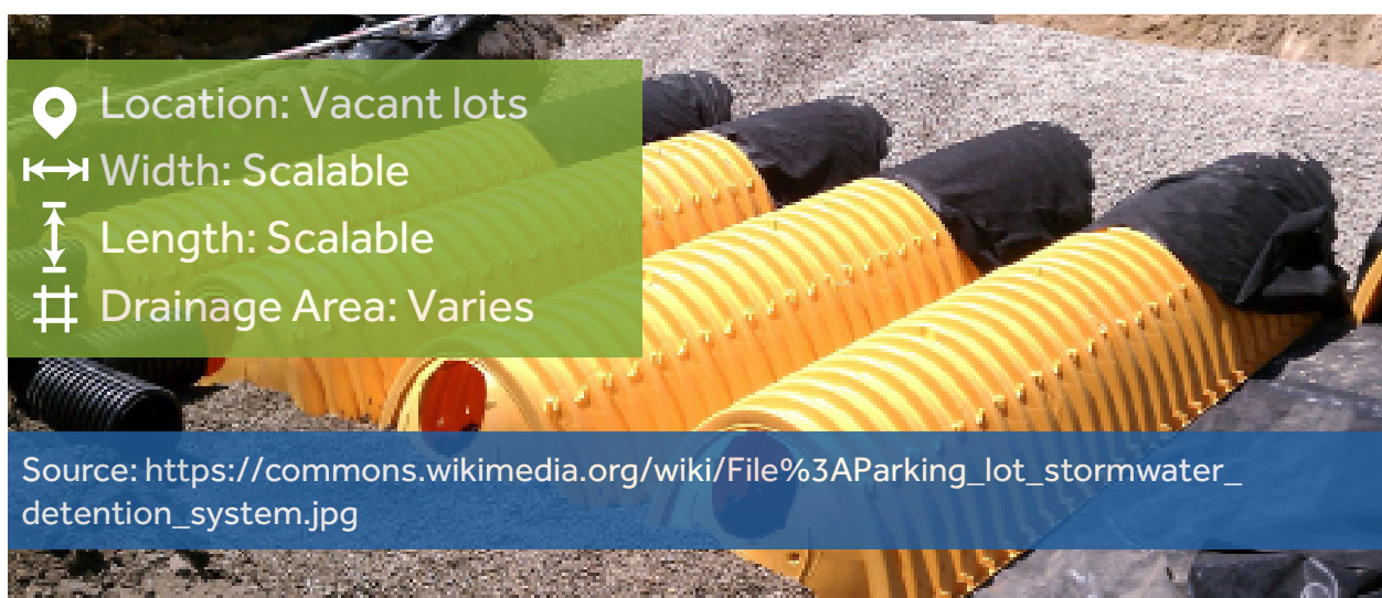
Figure 10: Underground storage chambers for stormwater
